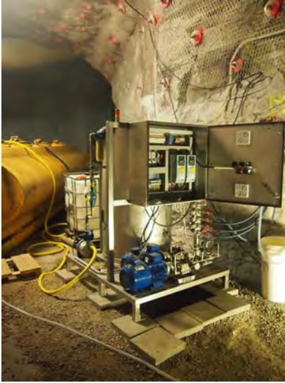
Pressurization system and water supply tanks
