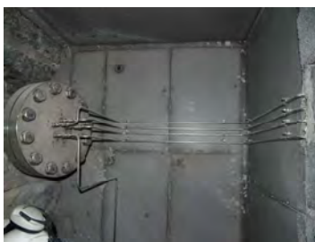
Pressurization pipes mounted onto the concrete backwall surface and passing through a flange of the rock lead-through pipes
