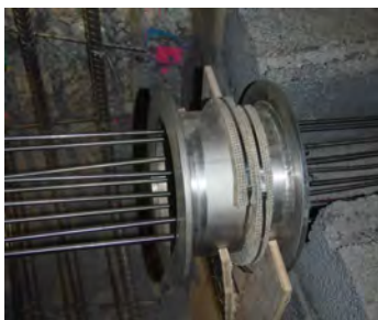
Wire flange for sealing of cables passing between filter layer and plug section I during construction
